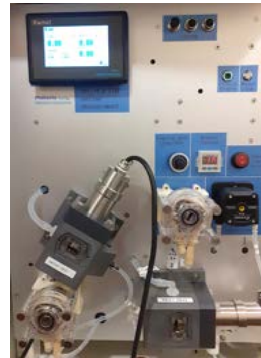
Nitrate Monitoring Station
